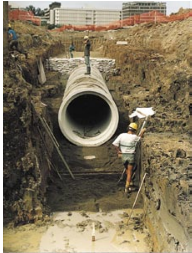
Rubber Ring Joint drainage pipes - note the trench construction to ensure a stable worksite.
