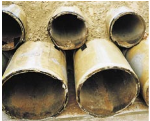
Pipes manufactured in 1920 at Loveday S.A. have been exhumed and reused in a culvert at the Gurra Road Project in S.A. in 2000.
