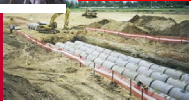
DRAINAGE, SOUTH EAST QUEENSLAND
