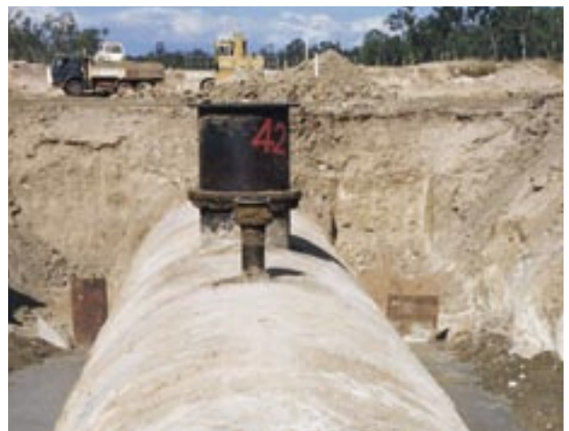
Air valve on 2700mm diameter skid ring joint pipe.
