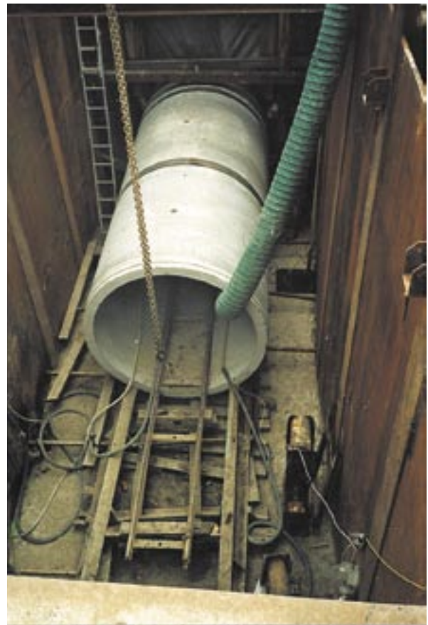
Stormwater pipes, jacking pit showing muck cart rail, air ducting and pipe joint type.
