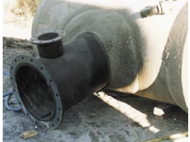
Cement lined mild steel off takes.
