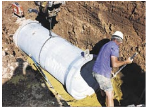
Preparing the bedding at the socket end of the pipe to be joined.
