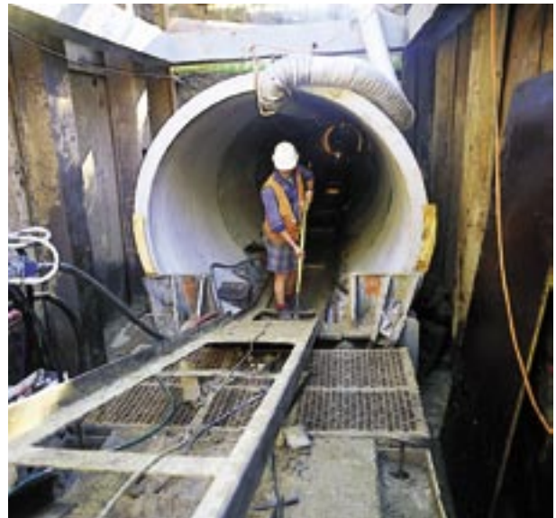
A typical jacking pipe installation, note air ducting and rail transport of spoil mat.
