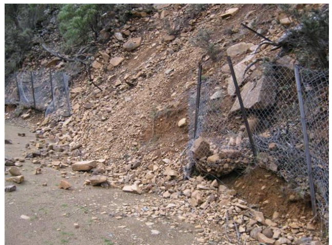
An existing single twist mesh (chain link type) low energy rock catch fence that has been destroyed by a rockfall event at the site
