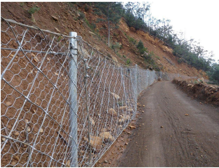
A number of rockfall events have taken place since the installation of the CTR-05-07-B rock catch fence. No maintenance to the fence has been required.
