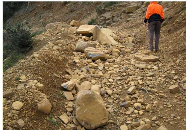
An example of the size and amount of boulders that have detached from the slope and impacted the access road prior to the installation of the proprietary catch fence
