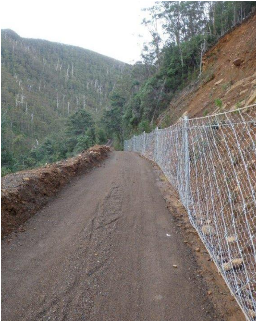
The track is now protected by the 100m long x 2m high rock catch fence. Note the combination of high stiffness High Energy Absorption (HEA) cable mesh panels and Double Twist (DT) mesh. This combination of intercept meshes means that during an impact, the deflection/elongation is less than that of a high tensile strength mesh with low stiffness. This makes the CTR-07-07-B fence suited for installations close to roads and infrastructure.
